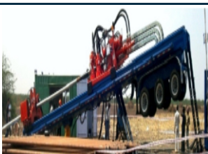
HDD Rig 6 American Augers DD 625 HDD Rig & Mud Cleaning System 300 Ton Pull Back Capacity HDD Rig Year Purchase 2012
