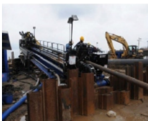
HDD Rig 5 American Augers DD 440T HDD Rig & MPR Drilling Fluid Mixing, Pumping & Recycling System mud Cleaning System Year Purchase 2012
